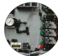
Pneumatic control systems
